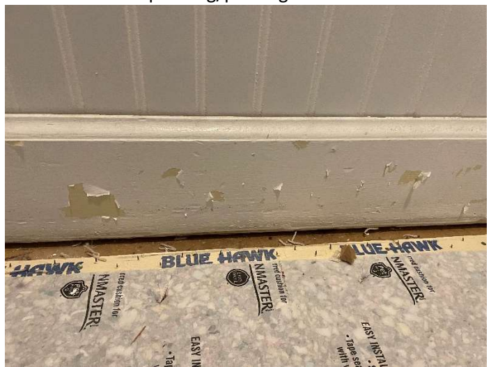
This is an example of the paint peeling from improper painting/priming.
